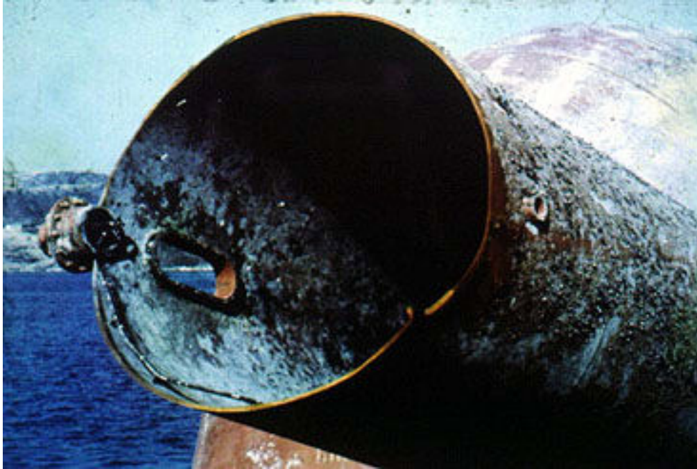
Figure 7 : The fatigue crack had propagated around the complete circumference of brace D6 from the defective origin of the hydrophone welded joint but no cracking to be observed emanating from the drainhole which is the same type of joint as at the hydrophone position.
